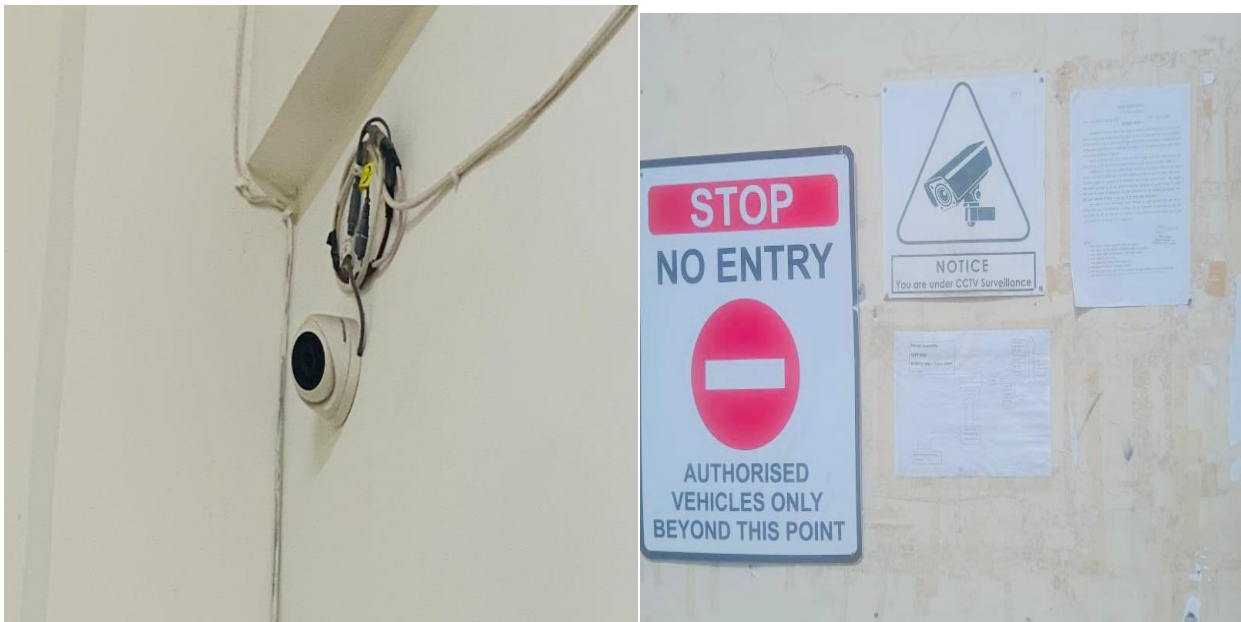
400 CCTV Cameras installed in the campus
